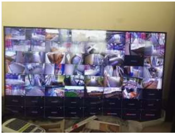
The security system with CCTV-cameras is up and working
